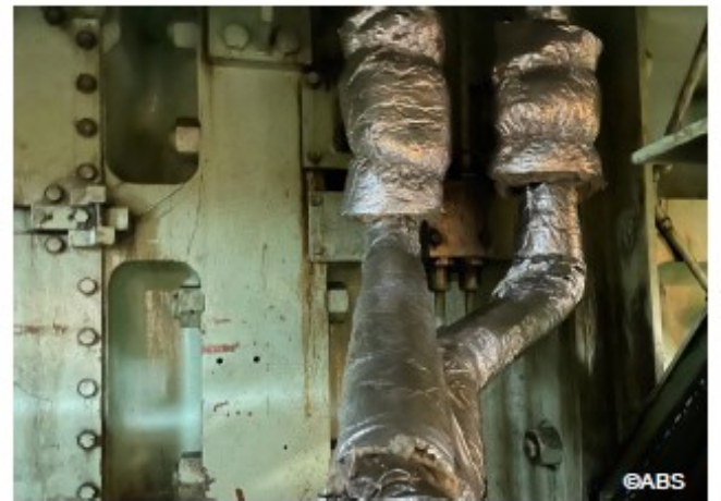
Fuel piping found without insulation – after
