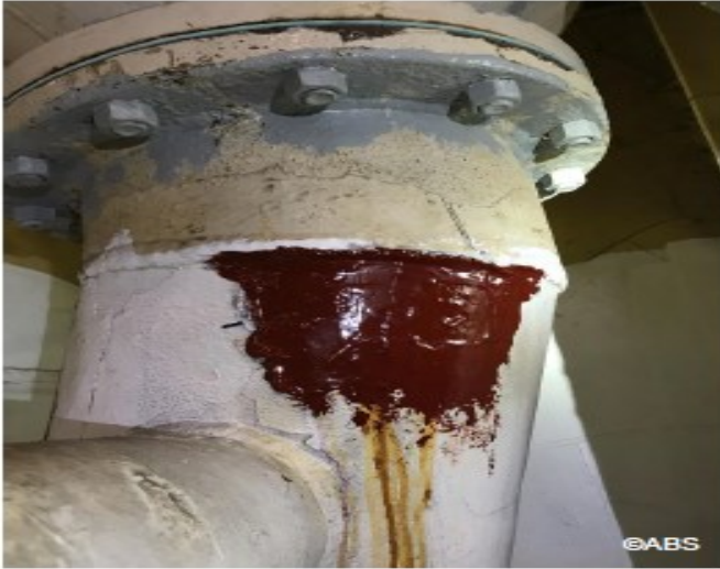
Ballast piping found with soft patch
