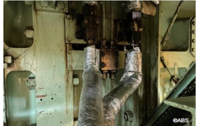
Fuel piping found without insulation - before
