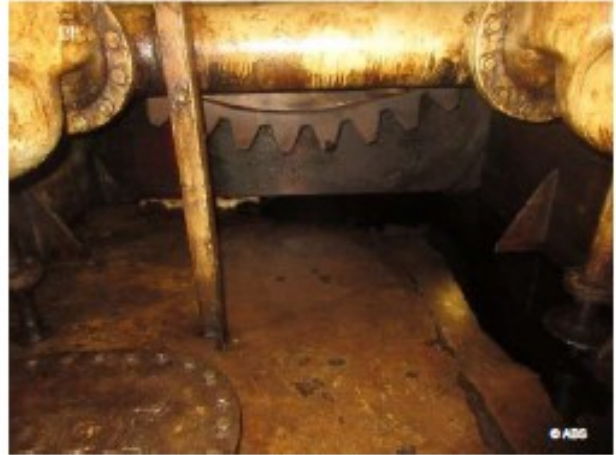
Cleanliness of engine room – fire hazard
