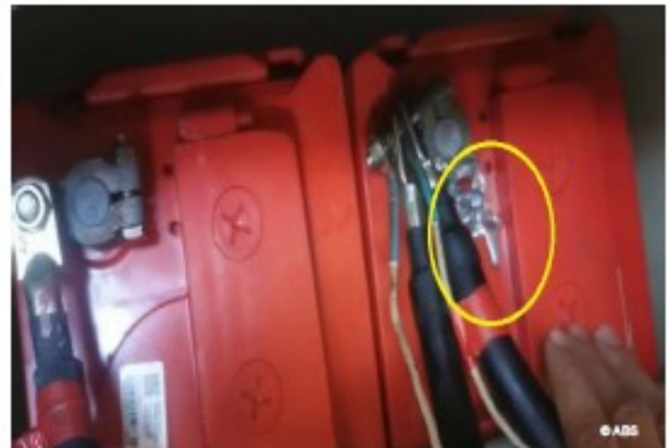
Lifeboat starter battery terminal connector broken
