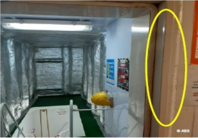
Engine room door gasket worn
