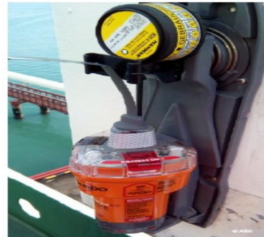
EPIRB antenna found deformed
