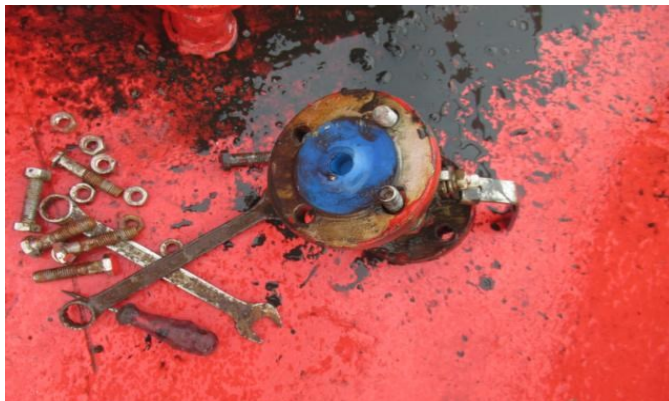
Bwt 2p Branch Valve Stuck with Plastic Cover
