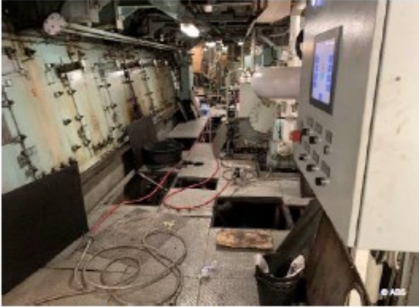
Cleanliness of engine room – before
