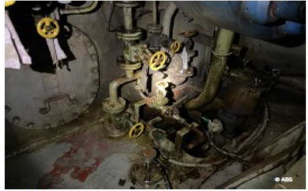
Cleanliness of engine room – fire hazard
