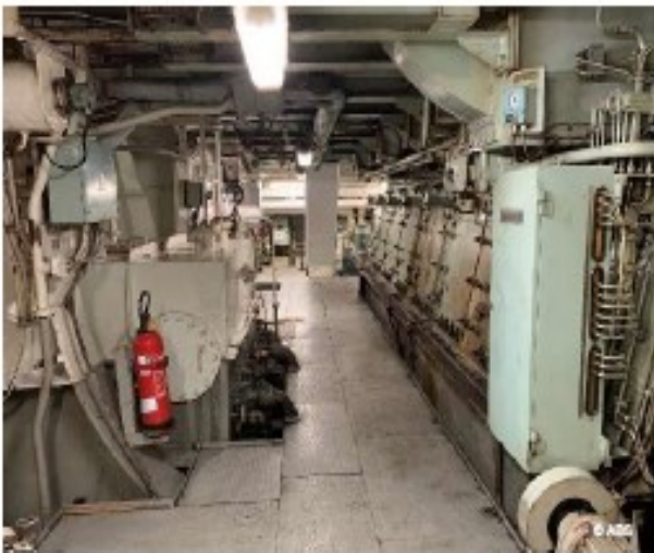
Cleanliness of engine room – after
