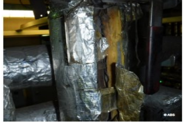
Damage to insulation on purifier piping
