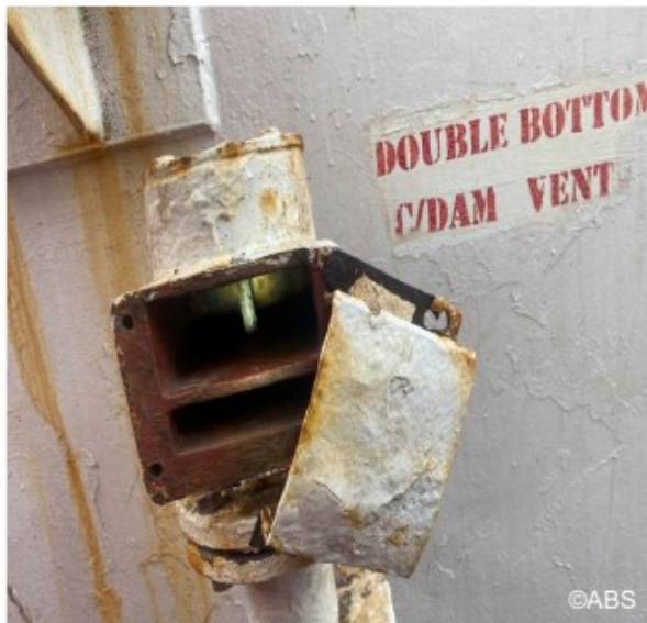
Ballast tank vent head disk missing
