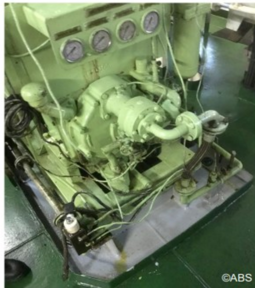
Oil leakage from main air compressor pumps
