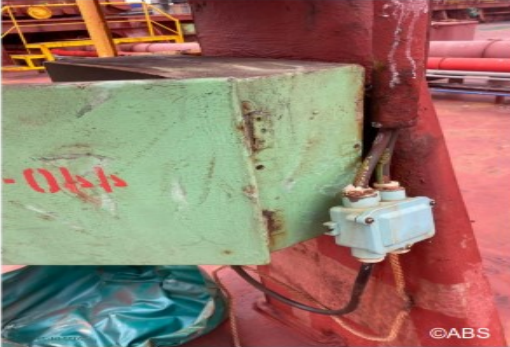
Unsecured junction boxes and cables on deck
